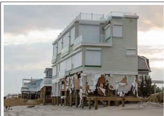
An example of a home damaged by Sandy. Is it substantially damaged when most of the structure was above the flood level?
