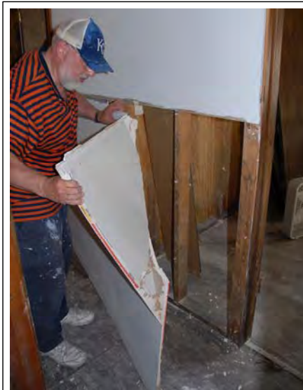
Property owners need to understand what is involved in cleaning a flooded house so it is safe to live in. Big Lake, MO, 2007.
